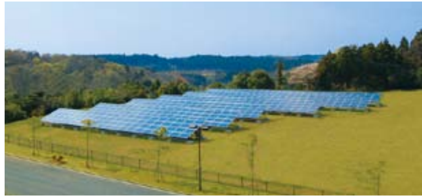
Solar power generation panels at the Kazusa Factory
